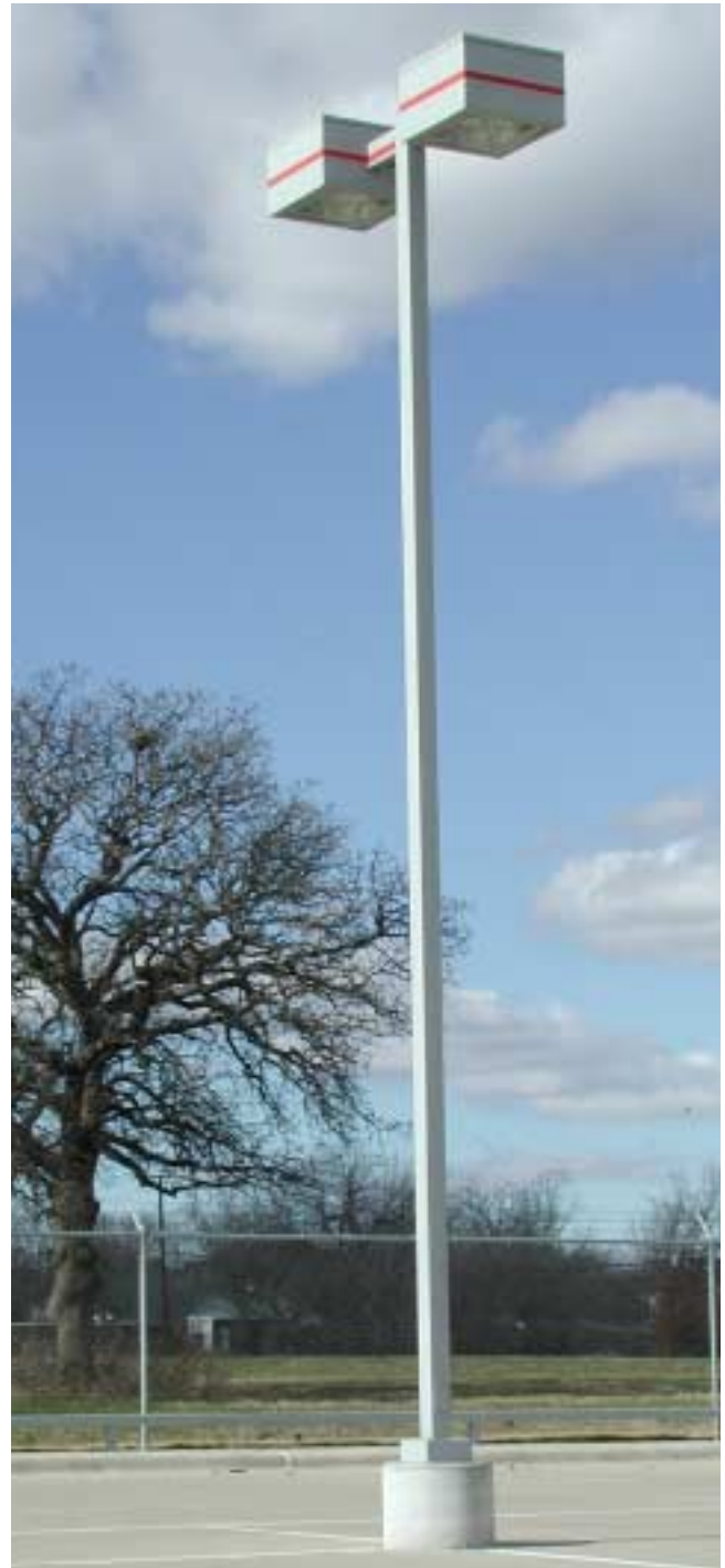
Figure 61 - Area Lighting Pole
