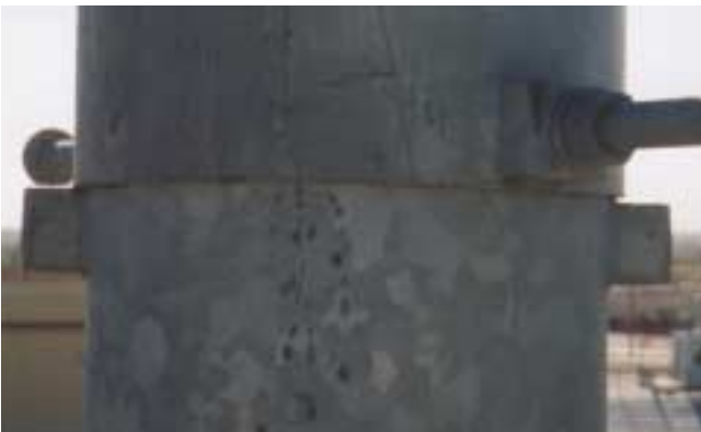
Figure 9 - Improper Slip Joint
